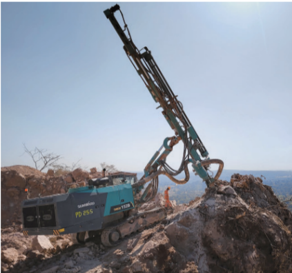
SWDE152B Slope operation
